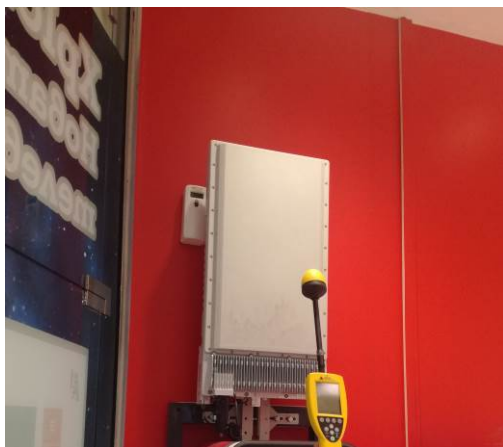
Figure 1. Picture of the fixed antenna on the inner wall of the premise
